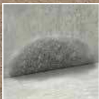
Leaking Areas of Voids i.e. Honeycombing
