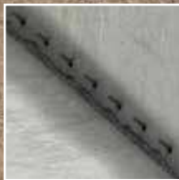
Leaking Construction Joints
