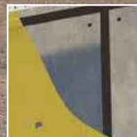
Leaking Compartment Membrane System
